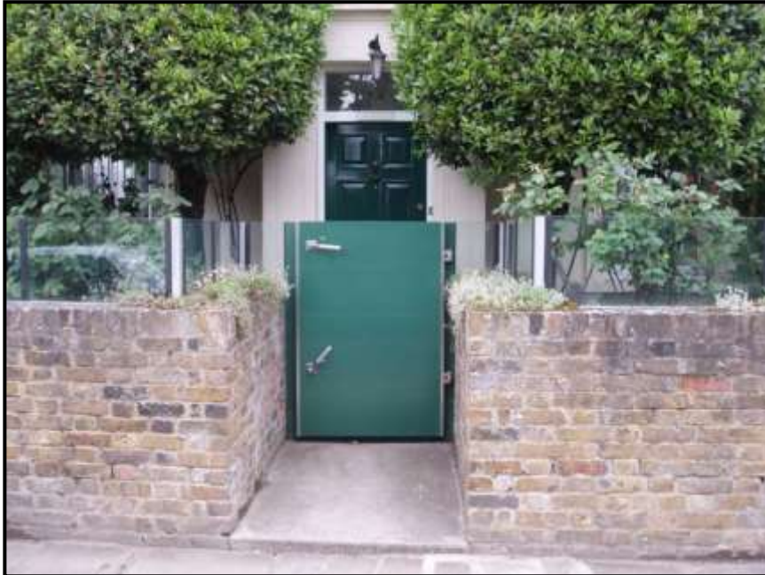
Figure 7-2: Permanent flood barriers
